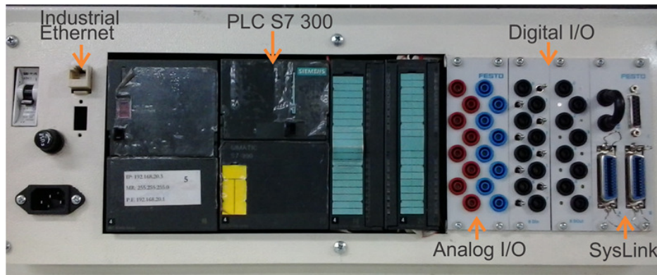
Figure 2. PLC s7 300 frame
